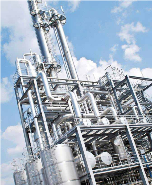
Potable alcohol plant – planned and realized by Vogelbusch
